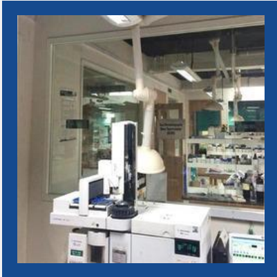
Lab Ceiling Mounted Extractor
