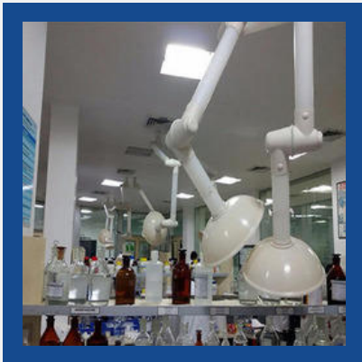
Top Ceiling Mounted Fume Extractor
