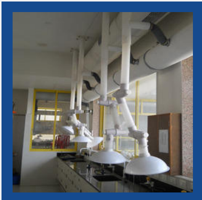
Polypropylene Laboratory Fume Extractor
