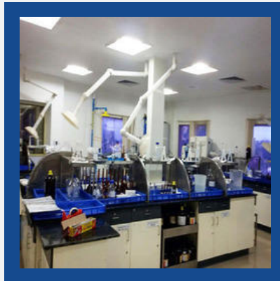
Chemical Ceiling Mounted Fume Extractor
