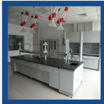
Laboratory Fume Exhaust System
