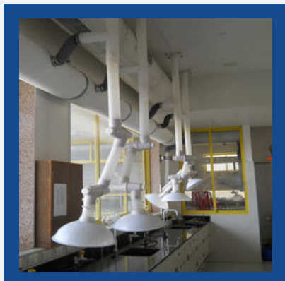
Fume Extraction Systems
